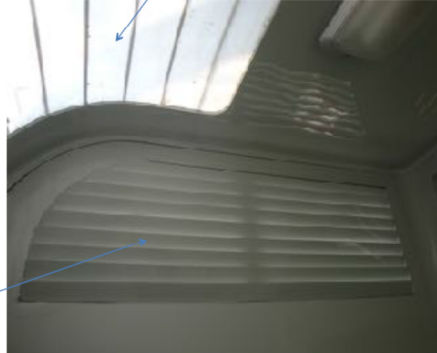
Natural air ventilation with provision of abundant Louvre arrangement
