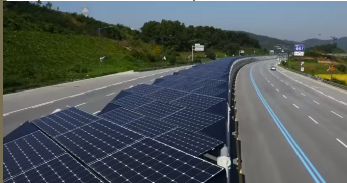
Solar roof top - 38 km cycle track
