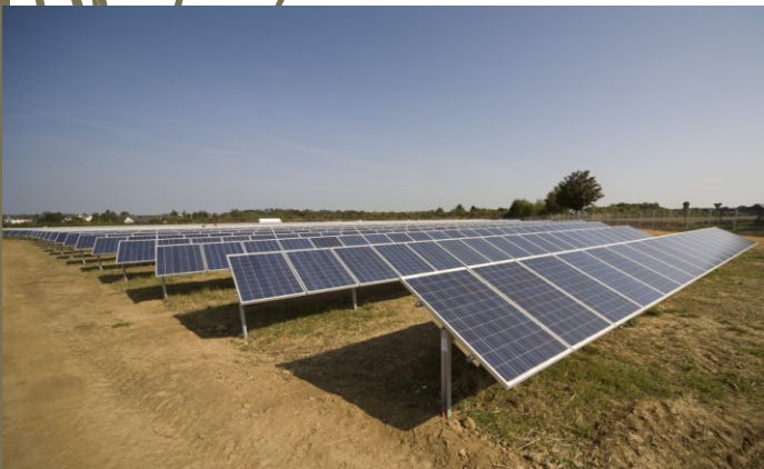
2MW capacity solar park
