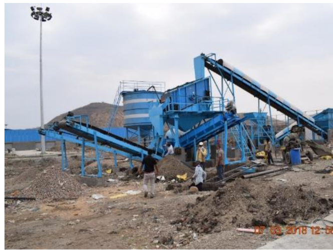
Waste Processing Plant
