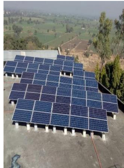
Devdharam Filtration Plant
