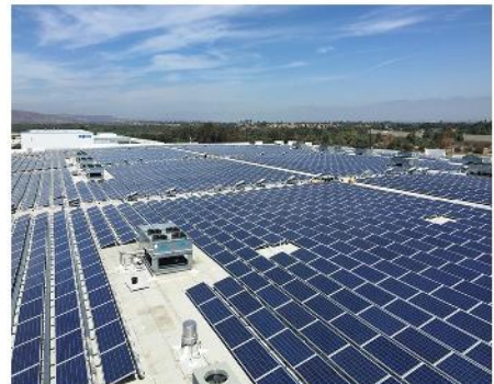
Solar panels on rooftop
