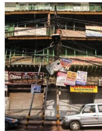
Over-ground wiring networks unsafe for all
