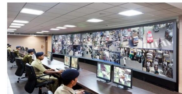
Emergency Response System
