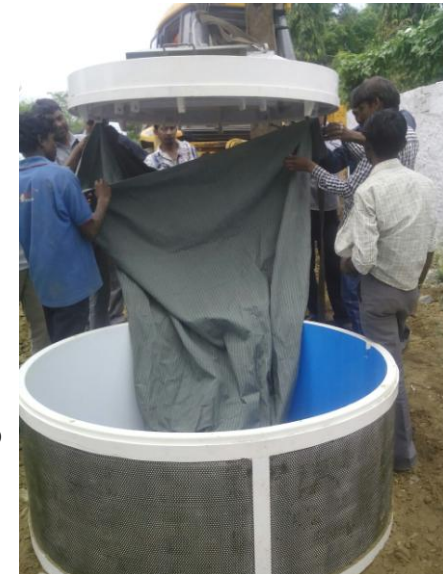
Already installed UG solid waste collector bins
